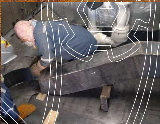
ACR 311 Cooling to Deck 3&4 FZ 3
